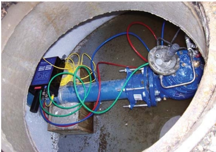
Figure 5: Flow Modulated PRV on Windsor Drive
