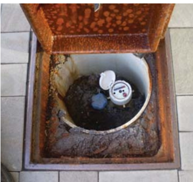
Figure 7: Commercial Water Meter Installed on Camp Street
